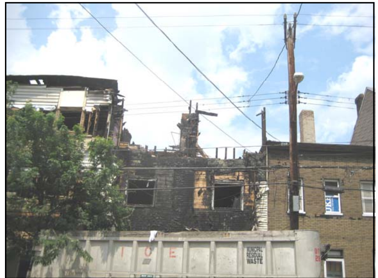
Fire damaged properties on Brereton Street from the November 2007 fire in process of demolition.
