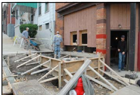
Pouring the cement patio for Café Lili. The café is slated to open in March.
