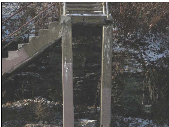
The supports for the steep staircase connecting Downing Street to Herron Avenue is crumbling.
